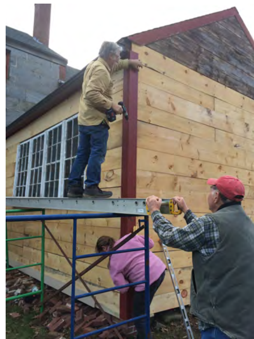
Ed Kavanagh assists carpenters Ron Stead and wife Mary with installation of new siding on the shed.
